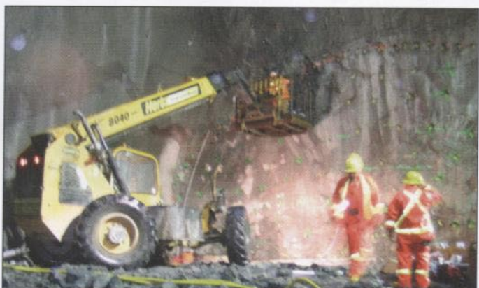
Drill+blast of the TBM assembly chambers and starter tunnels started in November
